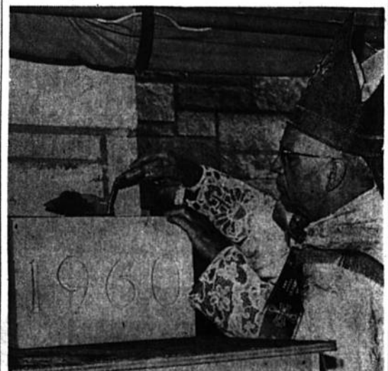
NEW FACULTY HOUSE: Archbishop Boland is shown laying the cornerstone for the new faculty house for the Christian Brothers at Queen of Peace High School, North Arlington. The ceremony was held on Aug. 15.
